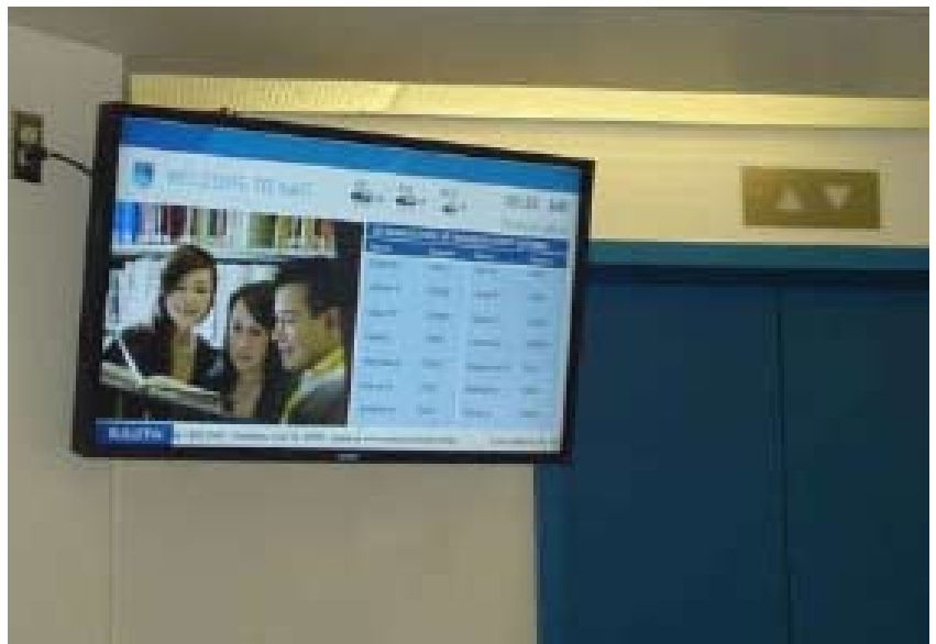
NAIT installed digital signage with up-to-the-minute class scheduling information in areas easily accessed by students.
